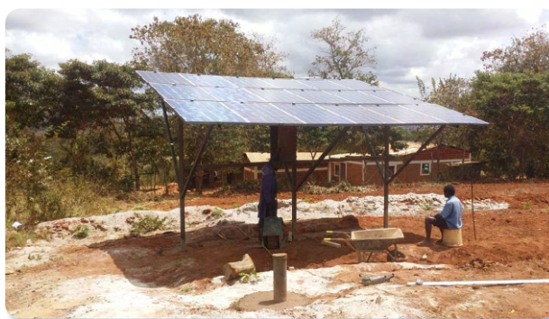
Image 8b: Image of solar system which delivers solar power for the irrigation systems from innovator Grekkon.
