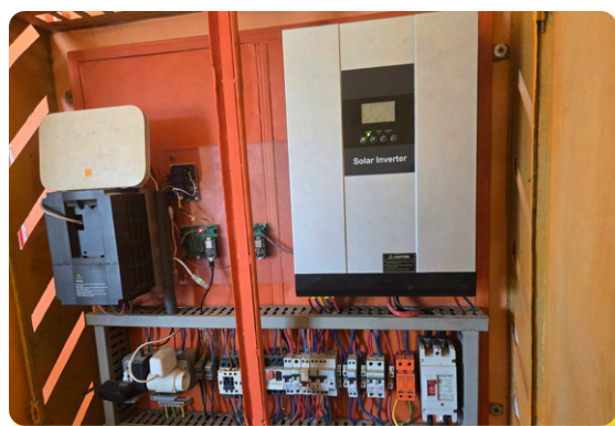
Figure 6b: Image of the converter inside the service center. All equipment runs on solar power, as the Walalma center has solar panels on top.
