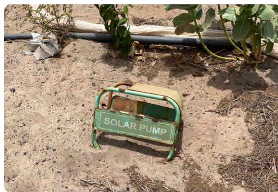
Figure 6b: Image of the solar pumps used for Ibriz' operations
